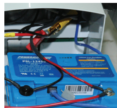
Fig. E (Battery terminals) Located in back on Ascend EL
